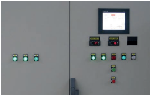
Fig. 6. View of the user panel in the electrical enclosure of the master PLC
